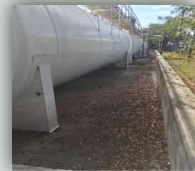
20,000-gallon Diesel ASTs, HART 21st Avenue Maintenance Facility
